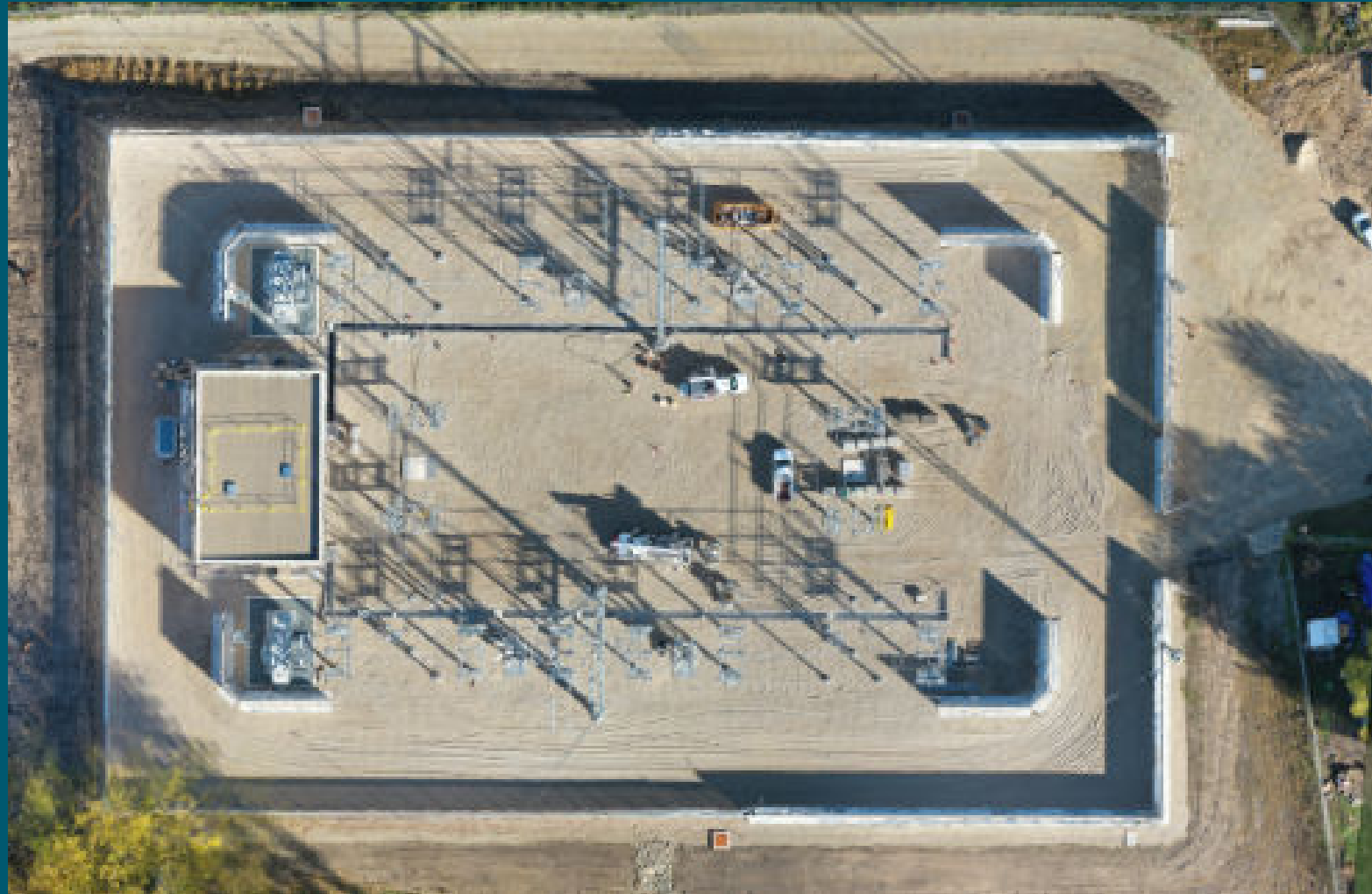
Description: Drone footage of the new electric distribution substation in SE Rochester
