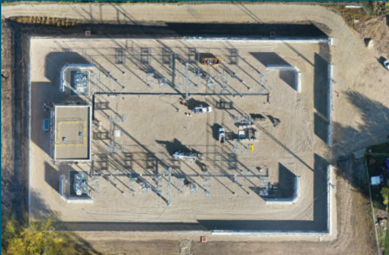
Description: Drone footage of the new electric distribution substation in SE Rochester
